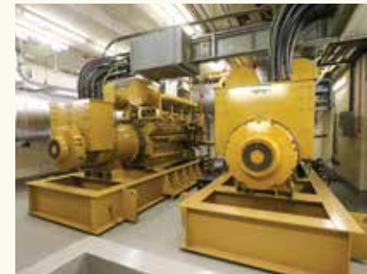
02 caterpillar generators, 100% back up
